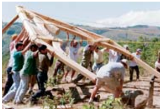
Above: The Kauai Timber Traming workshop last fall included round and square timber joinery.
